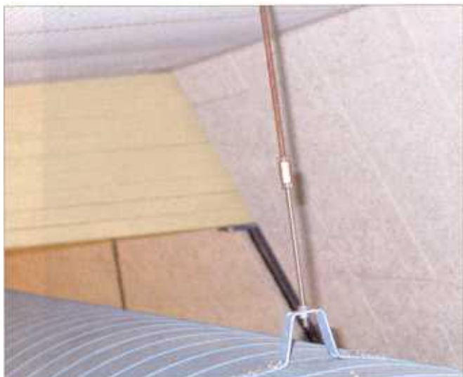
An air channel hanging on rusted and cracked stainless steel threaded bars. For unknown reason, the upper part is rusting stainless steel and the lower part is non-rusting galvanized steel (photo 2).
