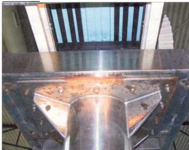
Rusted stainless steel AISI 316 construction, after six months of use (photo 3).
