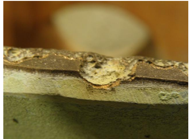
Close up erosion
