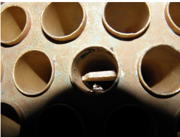
A lot of dirt in some tubes (close up)
