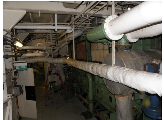
SB side evaporator
