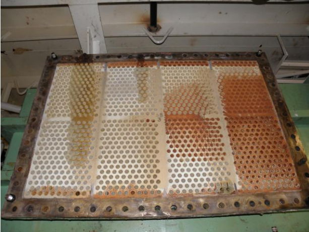
Tube sheet SB 3 no material delivery
