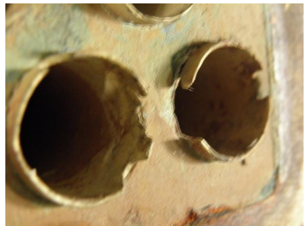
Tubes damaged (close up)
