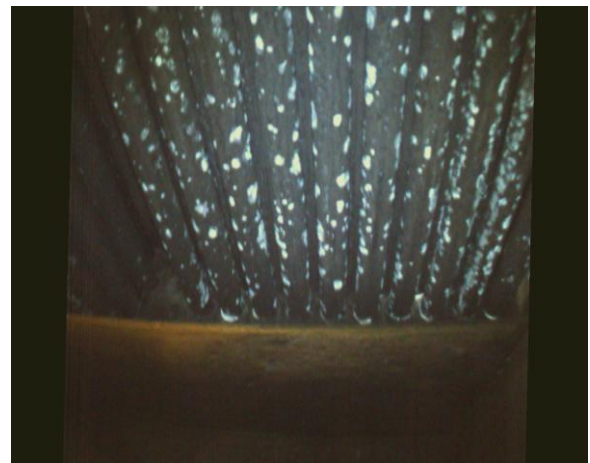
View under tubes SB
